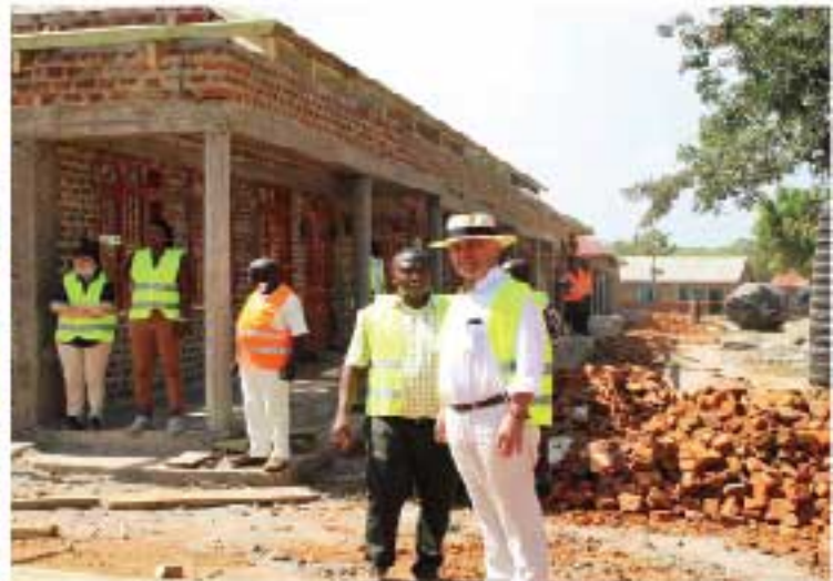
The Embassy of Iceland Team monitoring the progress of the construction works at Busiro Church of God Primary School
